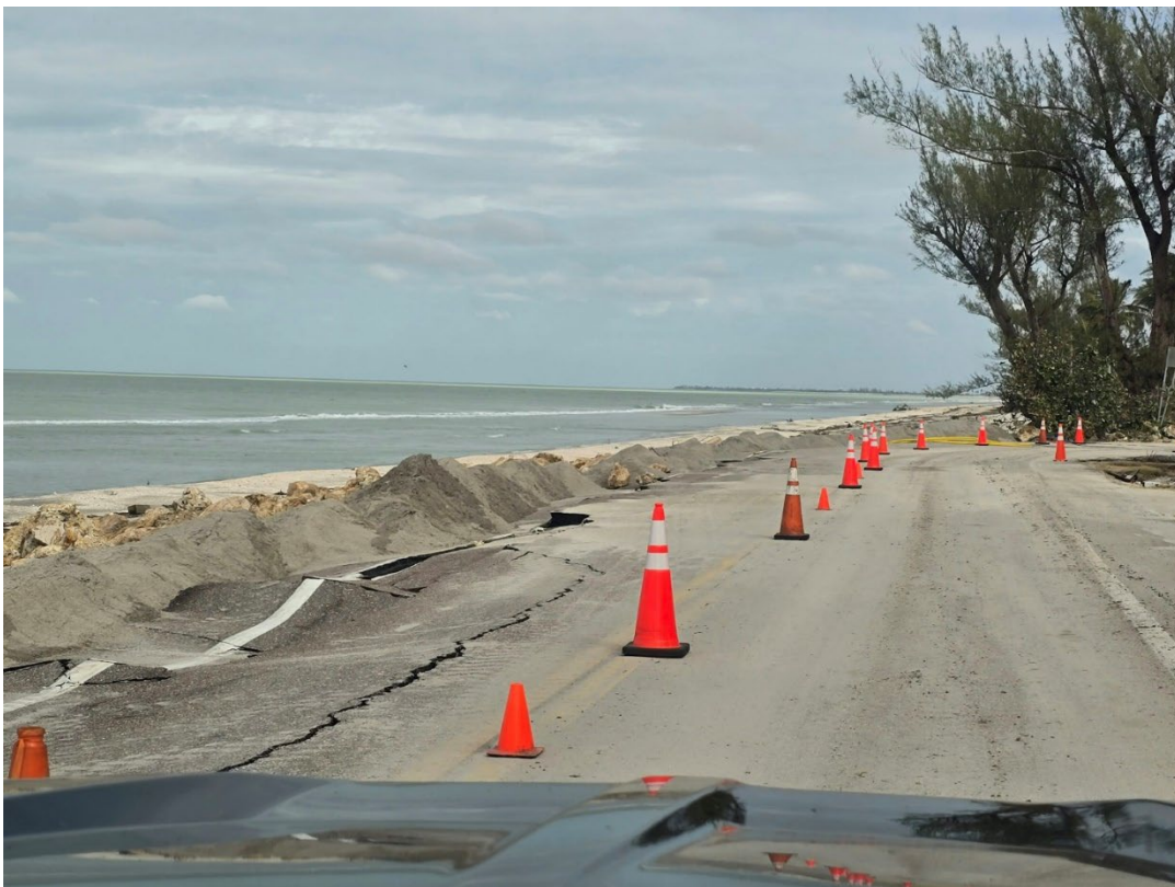
Figure 12. Impacts to Captiva Drive from Hurricane Milton (CEPD 2024).
