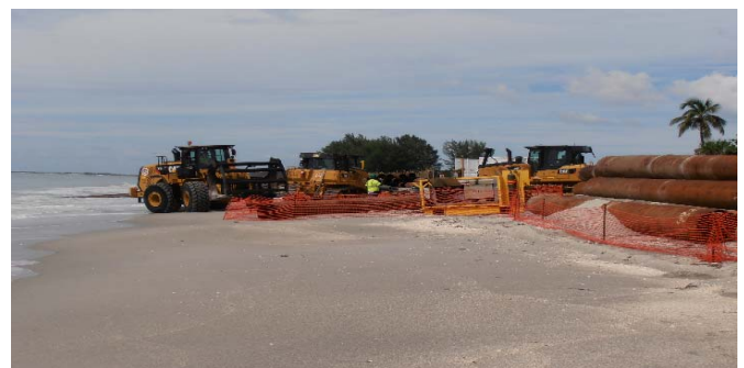
Bulldozers and pipe are staged at the beginning of the 2013-14 Captiva Island nourishment project
